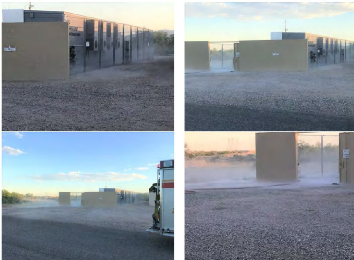
Figure 4 Photograph taken during the Surprise, AZ battery energy storage system incident, showing a white fog along the ground. Photograph from UL. 31
