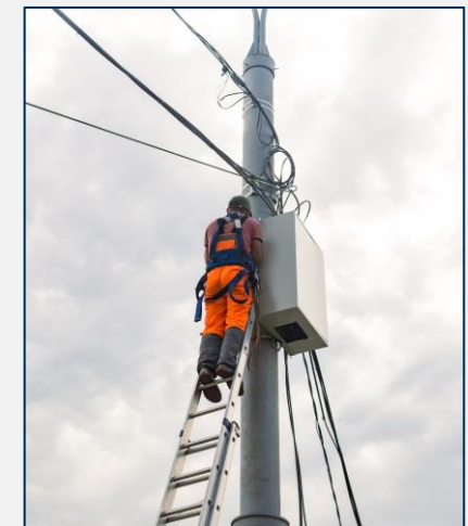
Figure 5: Utility Pole with Communication Lines
